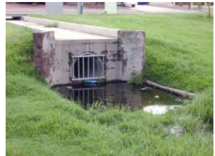
Figure 3 Keep roadside ditches and draining areas clear of debris so that storm water drains off easily.
